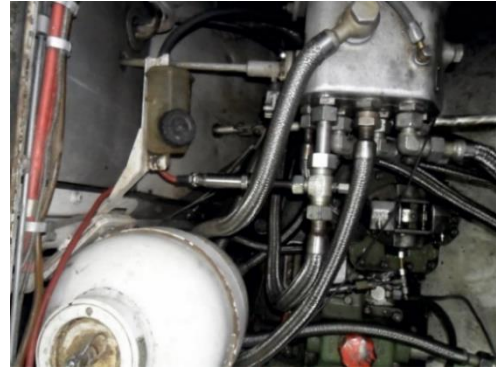
Fig. 15. Pressure gauge position.
